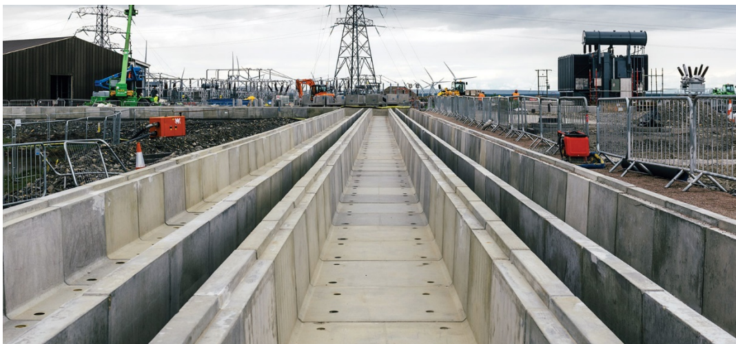
Figure 1: Typical pre-cast concrete cable troughs being installed for a power transmission project.
